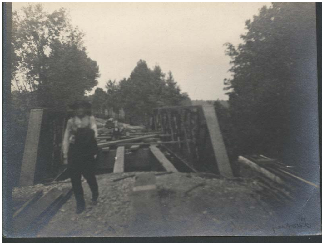
Figure 4. Alexander's Bridge, General view of trusses in position floor beams not yet in place, August 1907.
